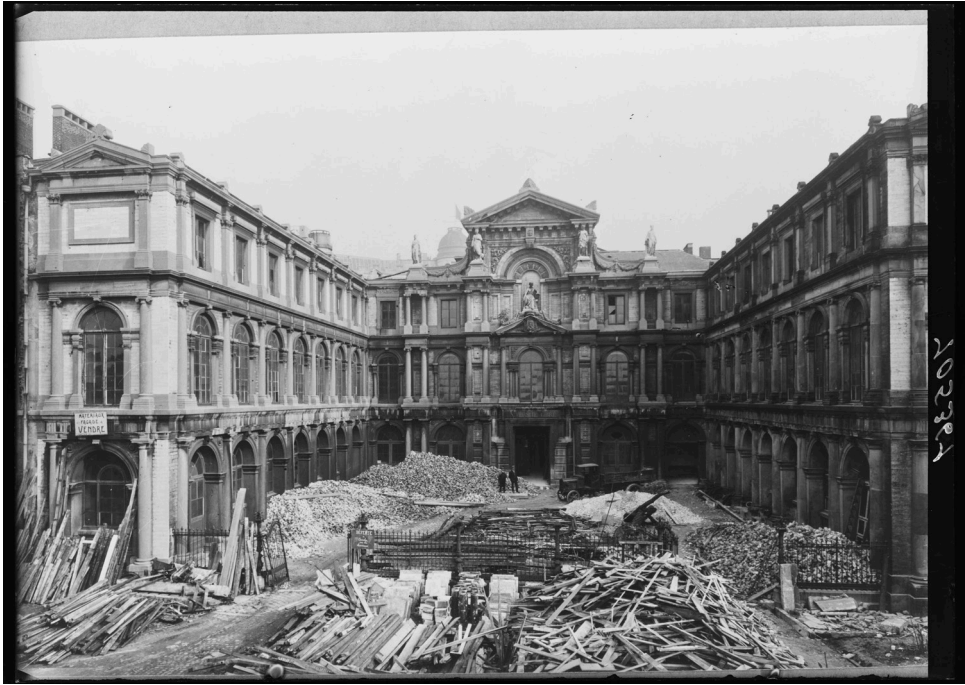
Demolition of Palais Granvelle in Brussels, 1928. (CC) BY 4.0 KIK-IRPA, Brussel, cliché A105361
